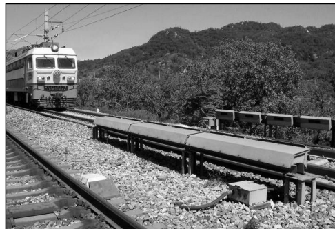
Figure 22. TADS® unit installed on Daqin line, China
